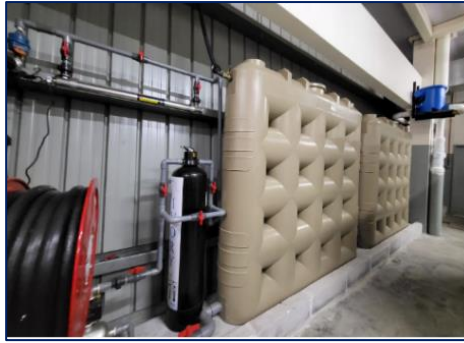
Figure 11: Rainwater Harvesting System
